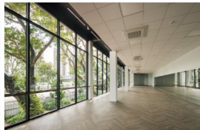
Indoor Hall The previously opaque façade was opened up with full height glazing replacing the brick infill within existing reinforced concrete frame. The former driveway and parking in front of this were also paved over to form a traffic-free connection from bus-stop to the indoor hall. Mature trees here were retained to provide shade and character, 2023. (Finbarr Fallon)
