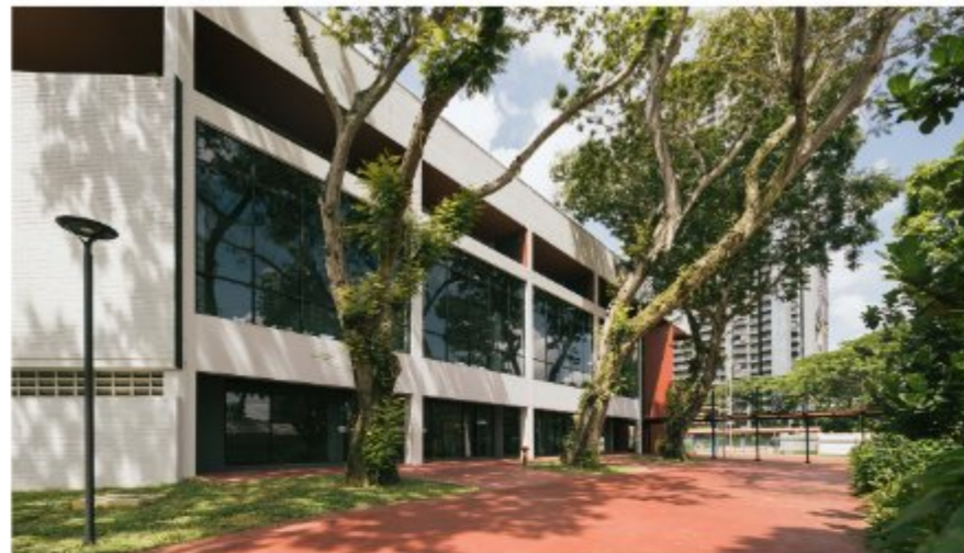
Indoor Hall The previously opaque façade was opened up with full height glazing replacing the brick infill within existing reinforced concrete frame. The former driveway and parking in front of this were also paved over to form a traffic-free connection from bus-stop to the indoor hall. Mature trees here were retained to provide shade and character, 2023. (Finbarr Fallon)
